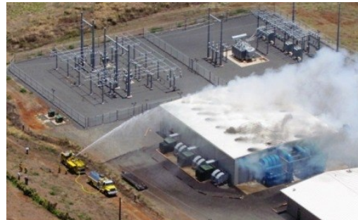
Fire at a battery energy storage facility
