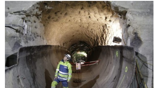
Rupture of the penstock/ tunnel at a pumped hydro plant under water pressure
